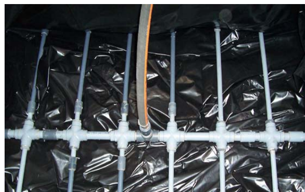
Fig. 3 Distribution manifold in disposal bag
